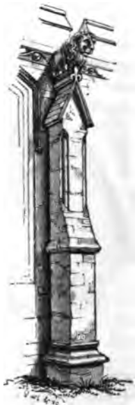
146. Over, Cambridgeshire. Buttress, with set-off and pediment, or gablet, with the angles of the upper stage chamfered.
